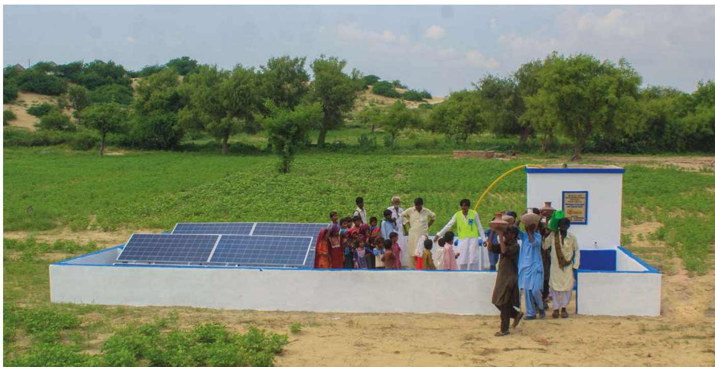
Villagers fetching water from Alkhidmat Solar Submersible Pump installed in a village in the District Tharparkar. Hundreds of families are benefitting from this project on a regular basis
