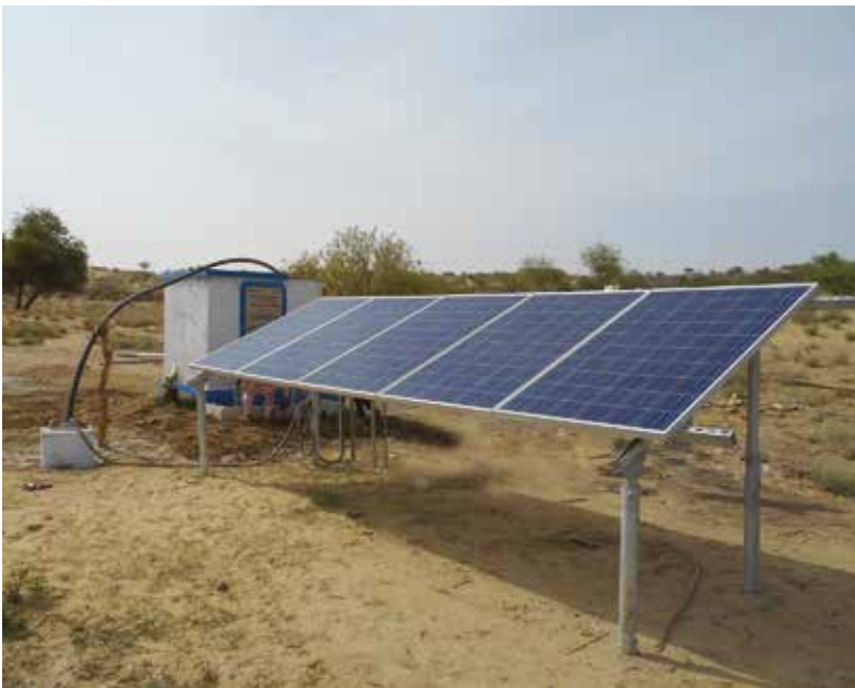
A Solar-powered Submersible pump working for the local community of Tharparkar, Sindh
