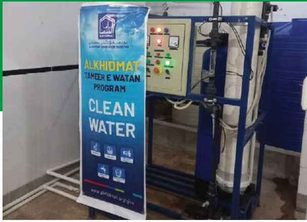
An operational view of a water plant.
