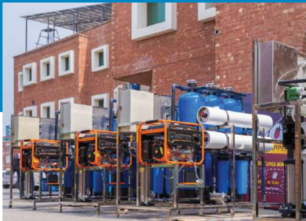
Water Filtration Plants stationed at Alkhidmat Complex Lahore.
