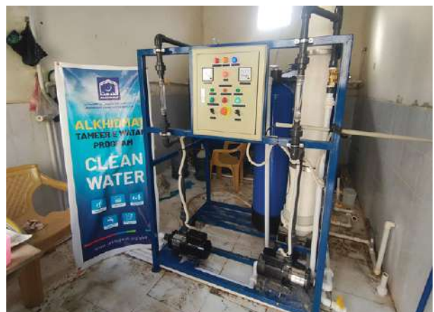
Water Plant installed under Alkhidmat Tameer E Watan Program.
